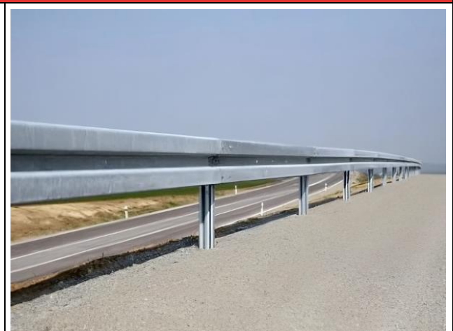
METAL BEAM CRASH BARRIER
