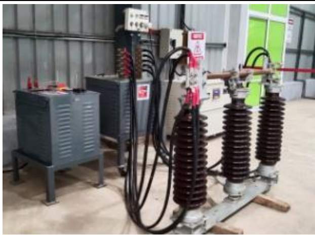
HV DISCONNECTOR STRUCTURE
